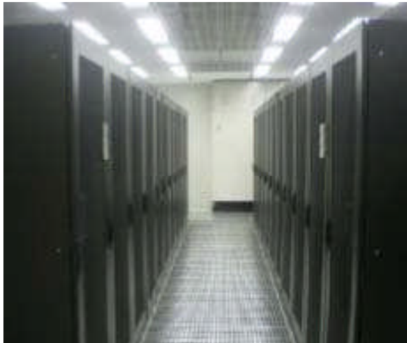
(a) Data center test room
