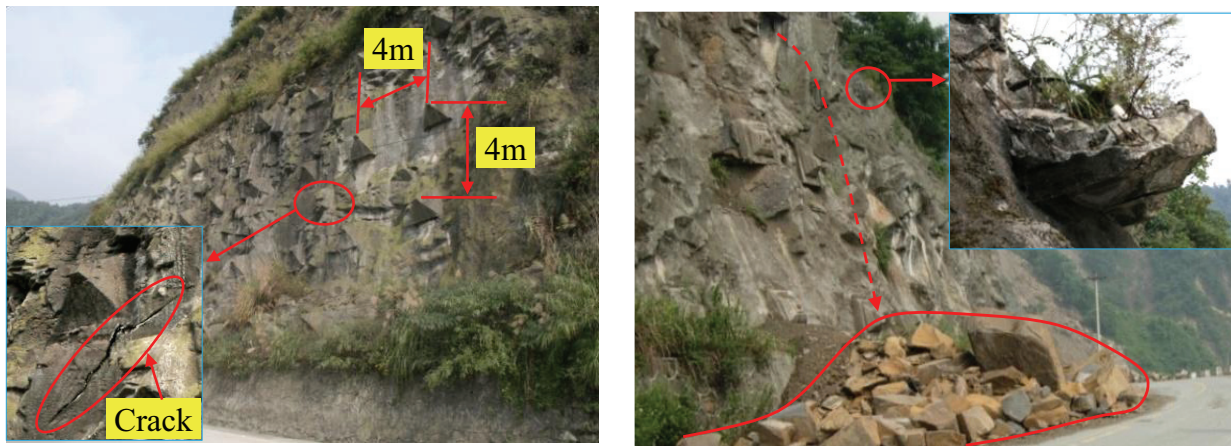
(a) visible crack nearby anchor head
