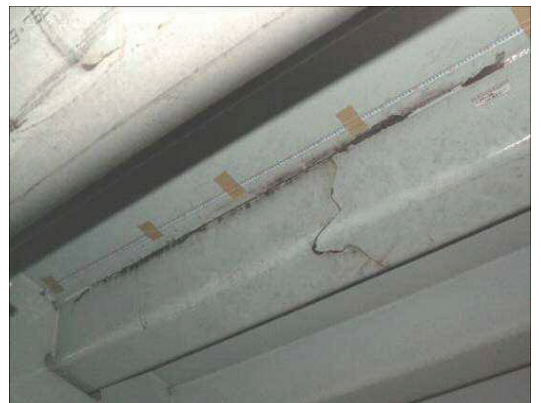
鋼床版Uリブのき裂
