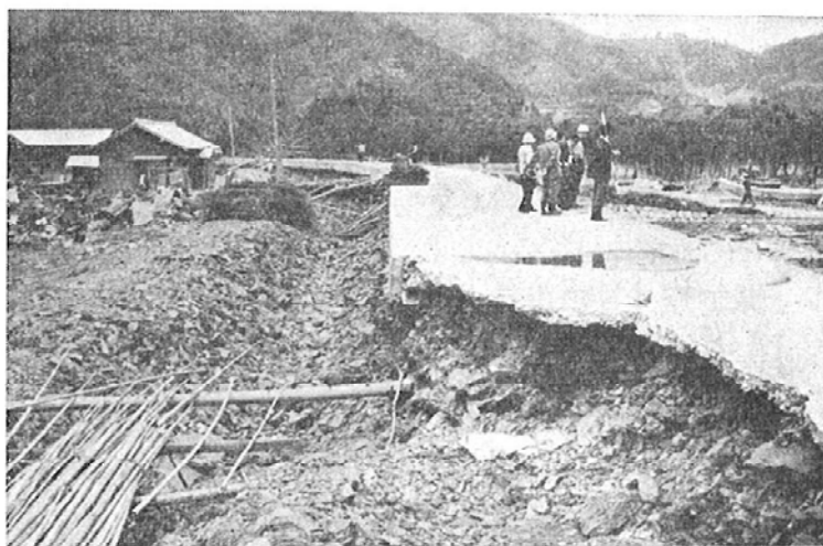
Plate 4. Failure of the sea wall at Ozuchi shown with a scoured ditch on the landward slope. Houses remained unscathed. A counter-tsu- nami grove is seen at upper right.
