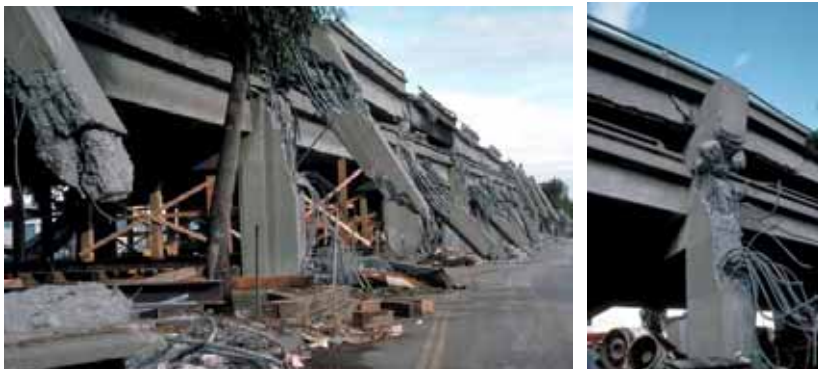
Figure 1.1 Cypress Street viaduct collapsed during the 1989 Loma Prieta earthquake. (Source: Wikimedia)
