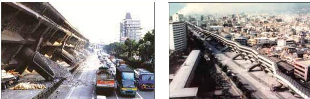
Figure 1.2 Hanshin Expressway collapsed during the 1995 Kobe earthquake. (Source: internet).
