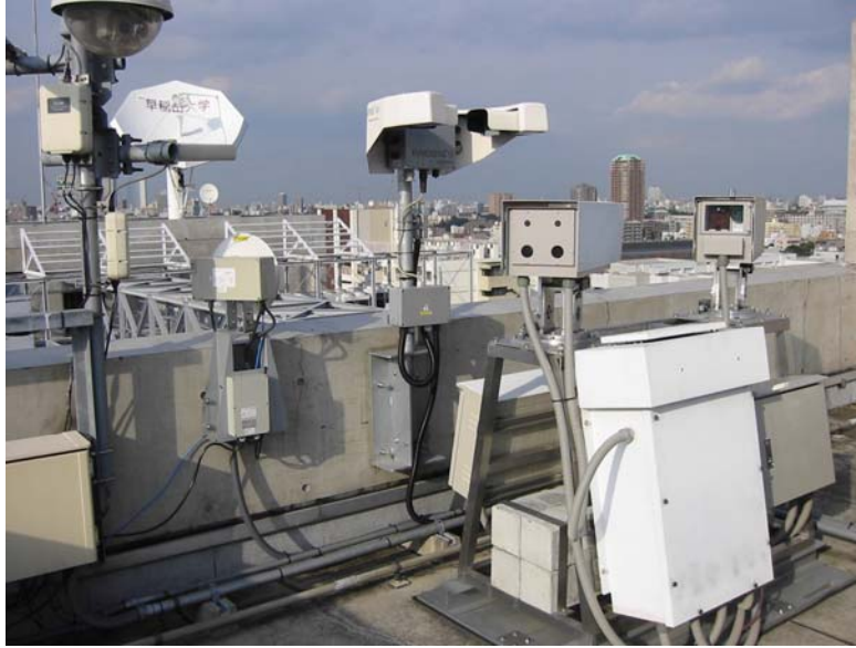
Figure 3.5: Devices setup on the rooftop of building 55 Okubo Campus
