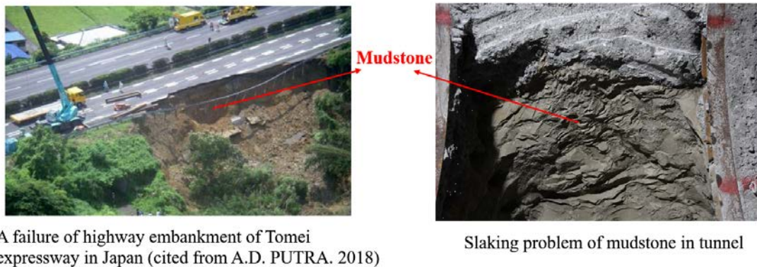
Figure 9-3 Slaking problem of mudstone in embankment and tunnel
