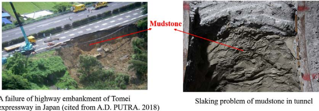
Figure 1-1 Failure of highway embankment and slaking problem of mudstone in Japan
