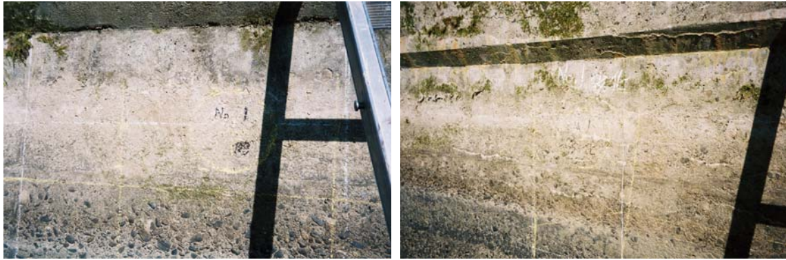
(a) No.1 (左：健全部，右：劣化部)
