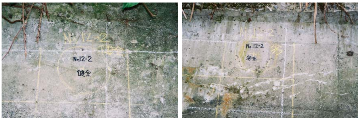
(f) No.6 (左：健全部，右：劣化部)
