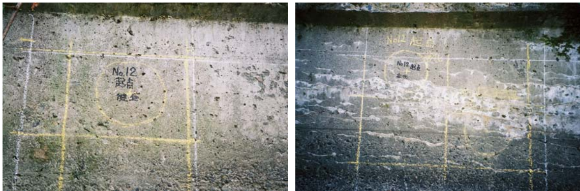
(e) No.5 (左：健全部，右：劣化部)
