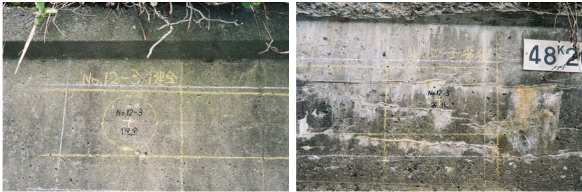
(g) No.7 (左：健全部，右：劣化部)
