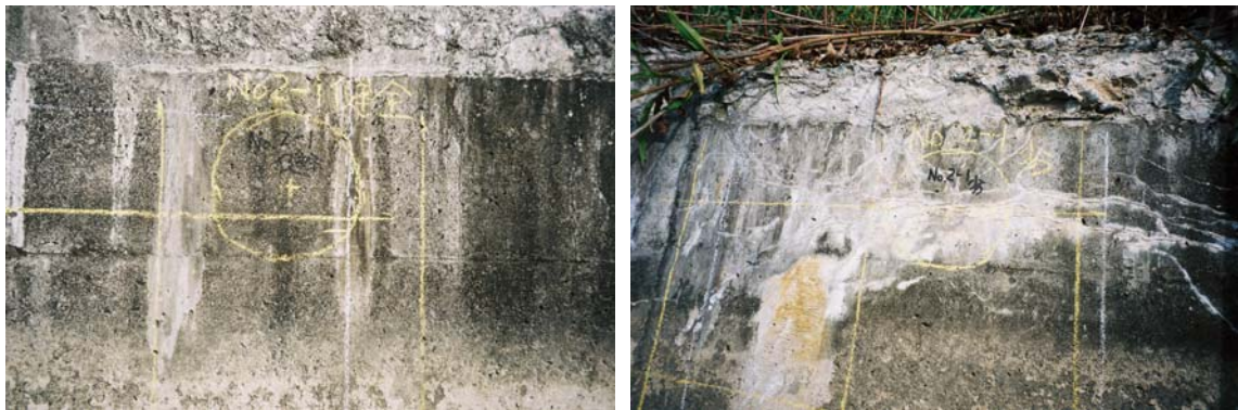
(b) No.2 (左：健全部，右：劣化部)
