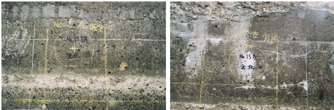
(h) No.8 (左：健全部，右：劣化部)
