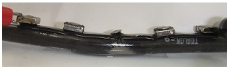
図 3.8 Broken MPW (disconnected)
