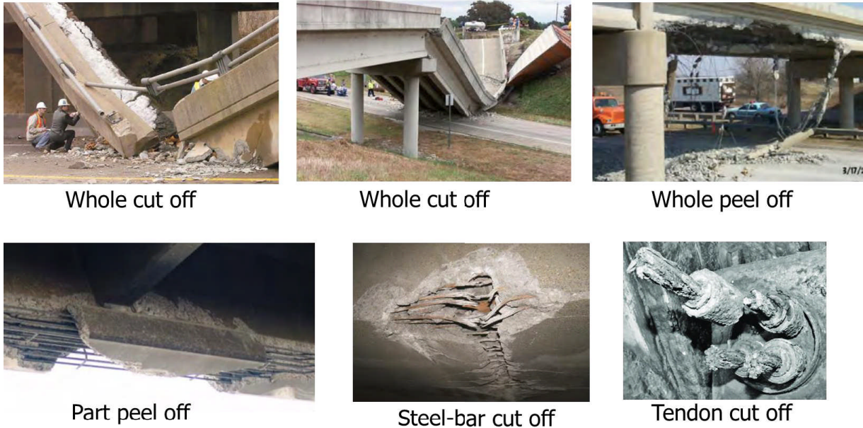
Figure 1.2. Types of damage form to the beam-like structure surveyed in the USA.
