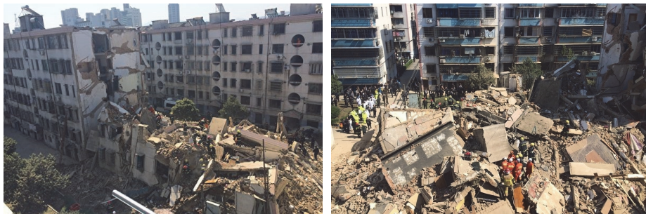
Figure 1-4 Collapse of an early 1990s commercial residential building in Fenghua, Zhejiang Province, 2014 (Source: Shi, 2014)
