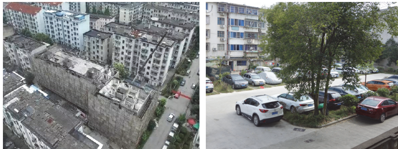
Figure 5-6 Jinshou No. 4 Building under reconstruction (left, source: BHUD) and new parking lot replacing old Building No. 4 (right, photo by author, 2018)
