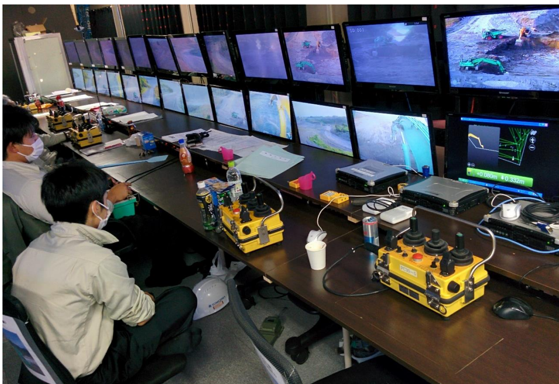
Fig. 1.8 Teleoperation room of an unmanned construction work ordered by Unzen Restoration Work Office, Ministry of Land, Infrastructure and Transport and constructed by Asunaro Aoki Construction Co., Ltd.
