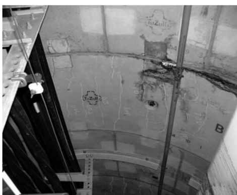
(a)天端のひび割れ
