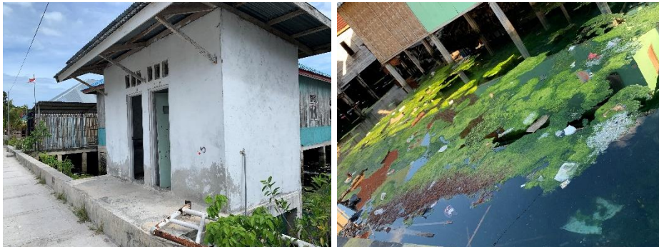
Figure 34 Abandoned public sanitation facilities (left) and contaminated waterscape (right)
